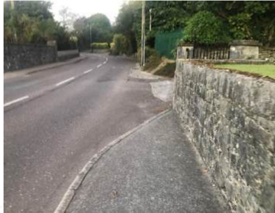
Photograph 9: View North East of St. Joseph’s Road North West Side Discounted Footway
